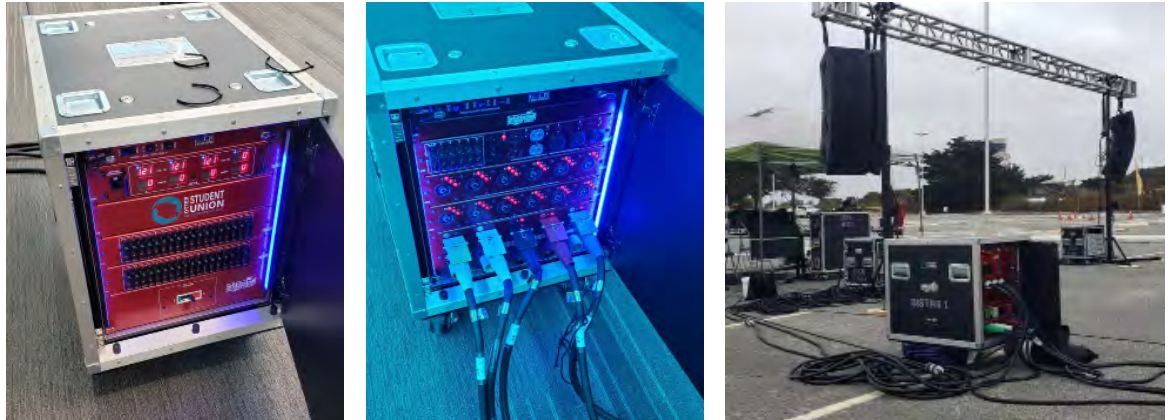
The new power distribution rack in use in the OSU Ballroom and its debut at the 2021 "Car-mencement".
